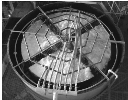
Fig. 3. Sarcheshmeh industrial plant flotation column
